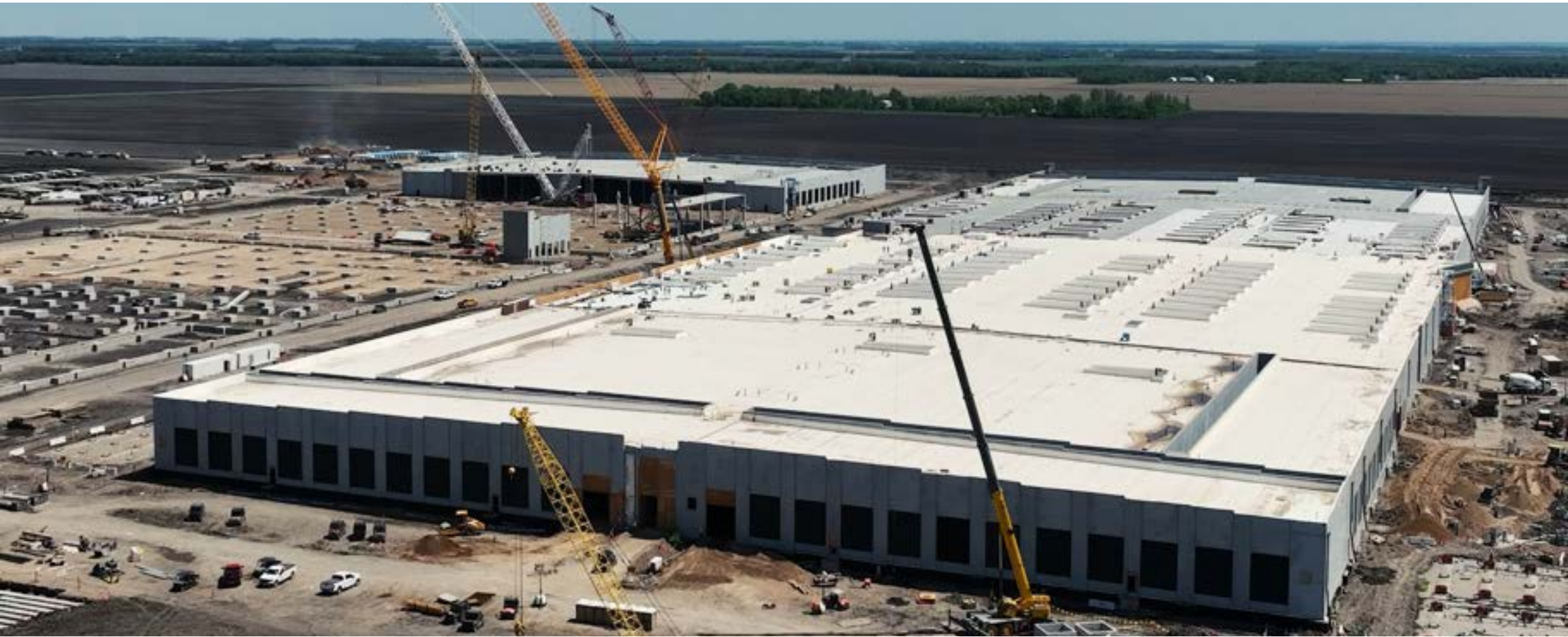
Building 1 - 150 MW - Standard Build (PF2 - 1)
