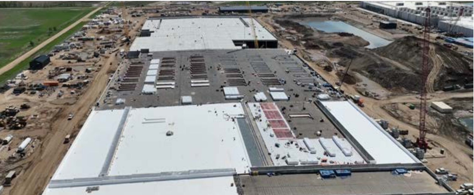
Building 3 - 150 MW - Standard Build (PF1-3)
