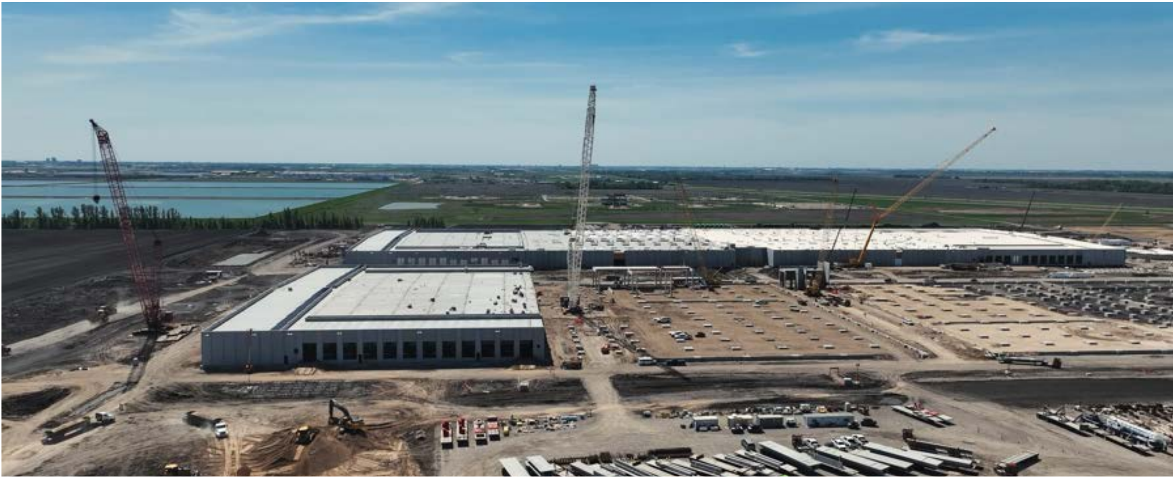
Building 2 - 150 MW - Standard Build (PF2 - 2)
