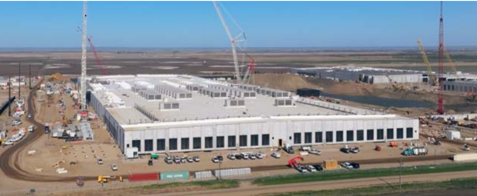
Building 2 - 150 MW - Standard Build (PF1-2)
