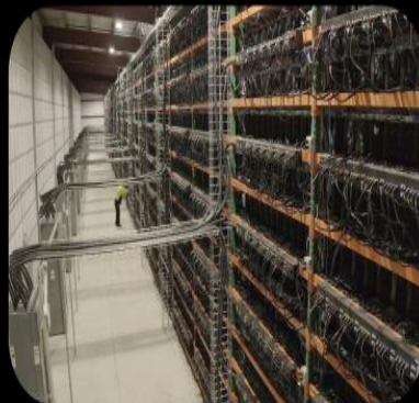
Jamestown, North Dakota Facility 100MWs
