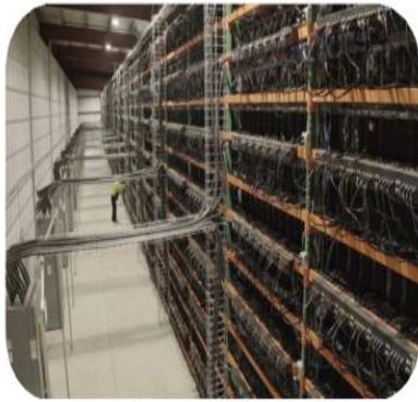
Jamestown, North Dakota Facility 100MWs
