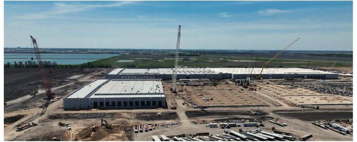
Building 2 - 150 MW - Standard Build (PF2 - 2)
