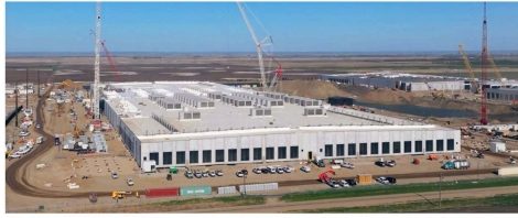
Building 2 - 150 MW - Standard Build (PF1-2)
