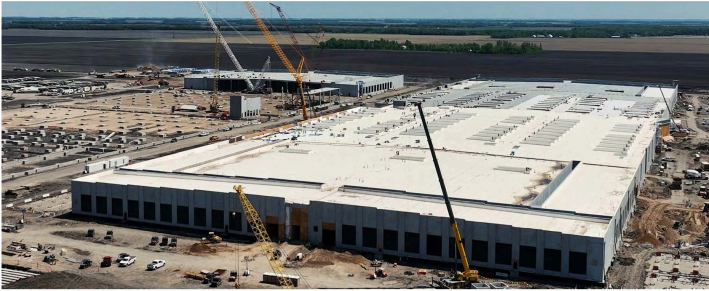
Building 1 - 150 MW - Standard Build (PF2 - 1)
